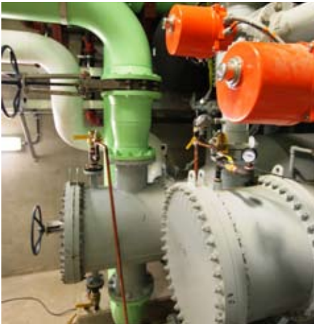
Southeast False Creek District Energy System photo courtesy City of Vancouver
